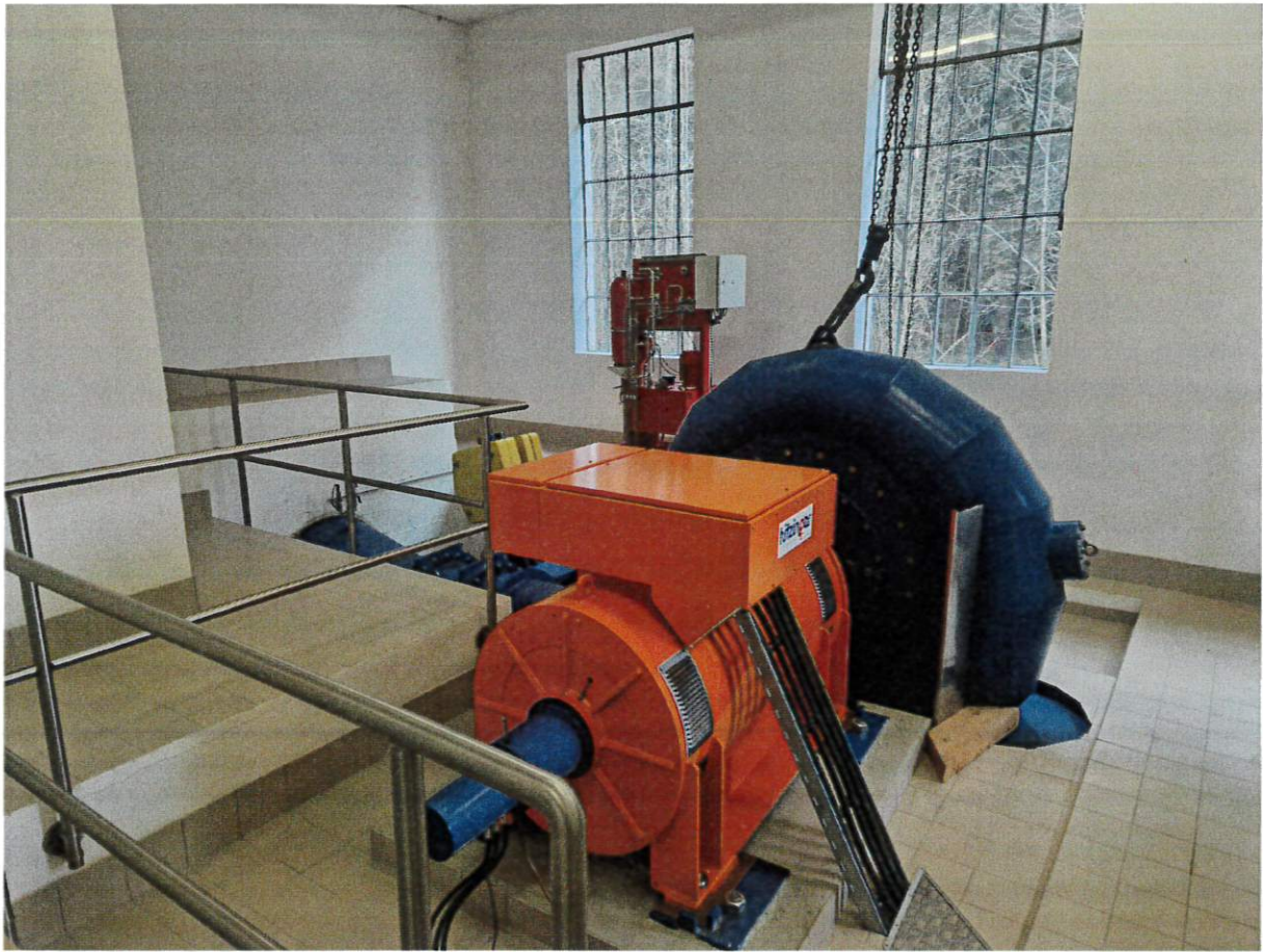
Francis – Diagonal Turbine 230 kw
